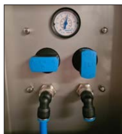
Connection on compressor
