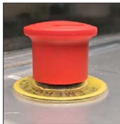
"Emergency" button pressed
