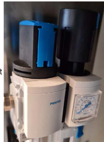
Shut-off valve compressed air in closed position
