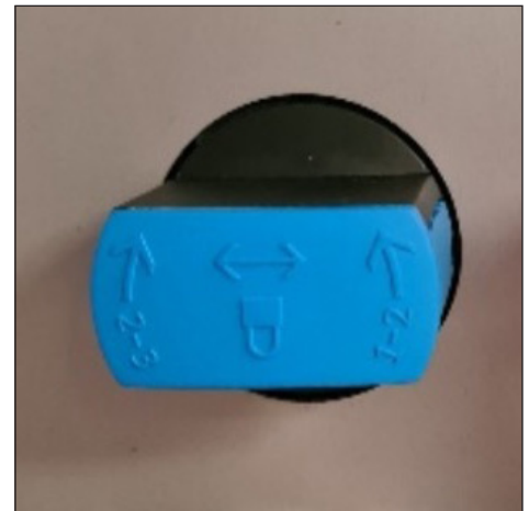
Compressed air valve in open state
