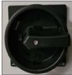
Main switch off
